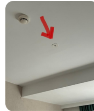
Example of a presence sensor found in our rooms.
