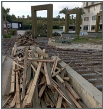
Unused Wooden Materials
